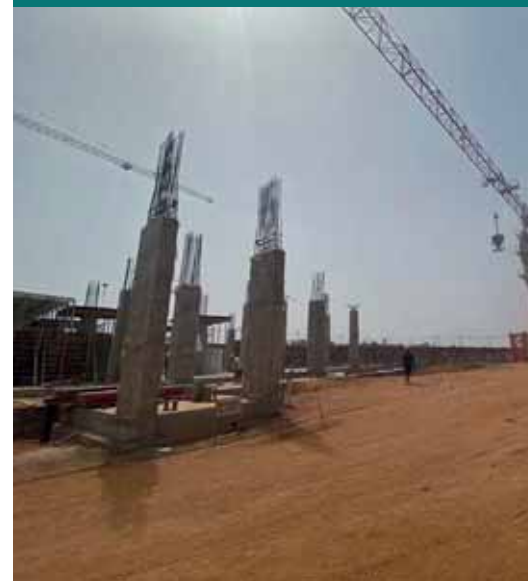
Above: Construction of the African Medical Centre of Excellence (AMCE) goes ahead in Abuja
